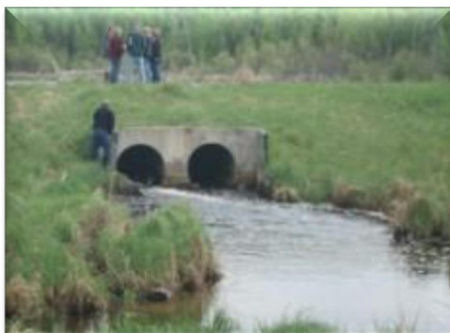
Pigeon Lake outlet before project.
