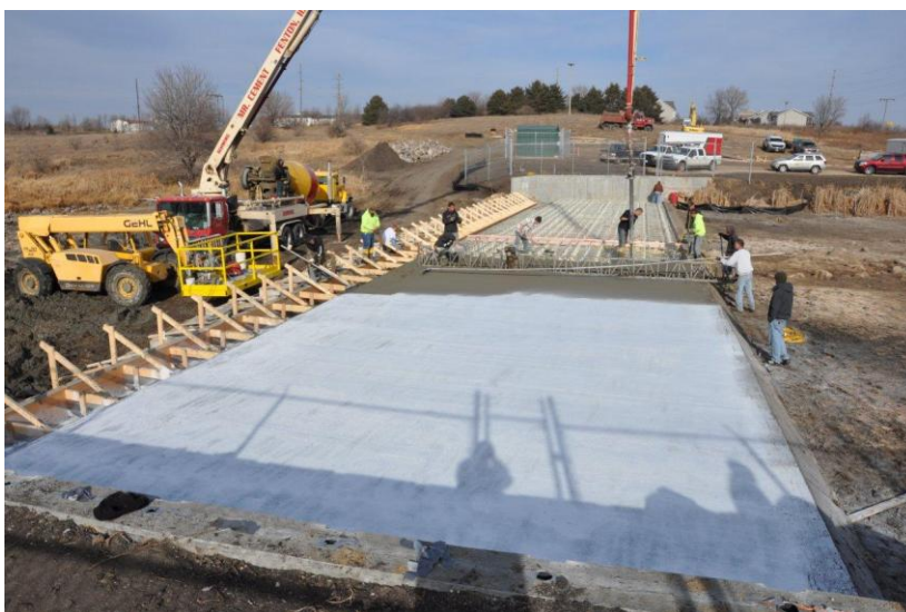
Electric barrier construction on Lower Gar outlet (Spirit Lake/Okoboji chain of lakes)
